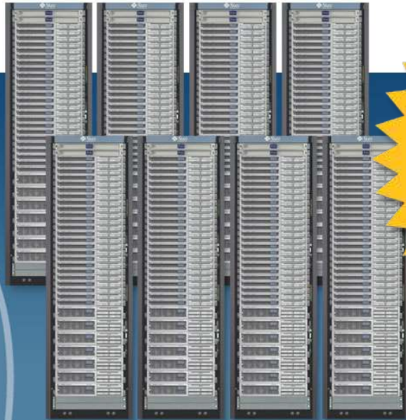
1,000 CPU Cores Total (8 Racks, 250 Sun Fire X4100 Servers)
